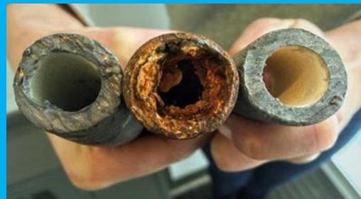
A lead pipe, a corroded pipe and a pipe with protective orthophosphate coating. Photo: USEPA
