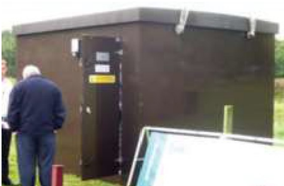
Figure 3 Typical orthophosphate dosing unit
