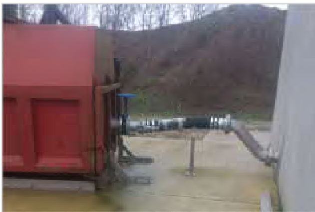
Figure 19: Enniscorty WwTP Dewatered Sludge Storage
