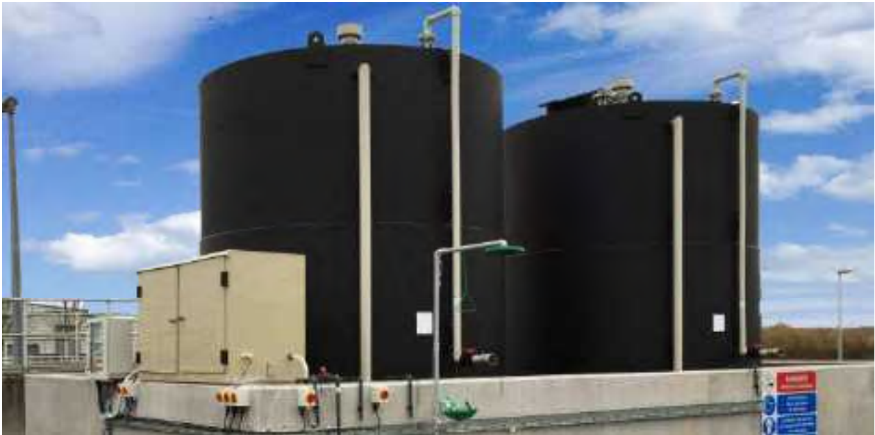
Figure 17: 2 no. 20m 3 tanks installed at Bunlicky WwTP (courtesy – Silotank)
