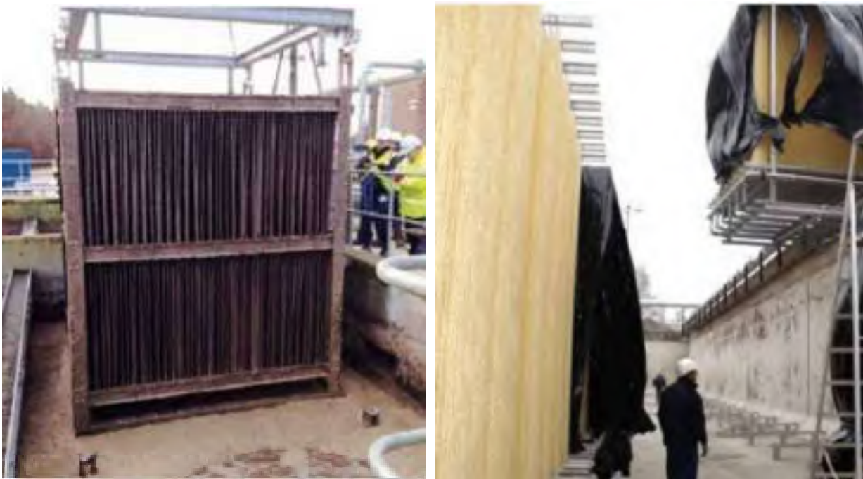
Figure 11: Example of IFAS frames and textile curtains (courtesy of Eliquo Hydrok)
