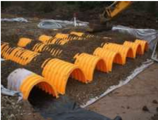
Figure 27: StormTech Storm Storage Tank
