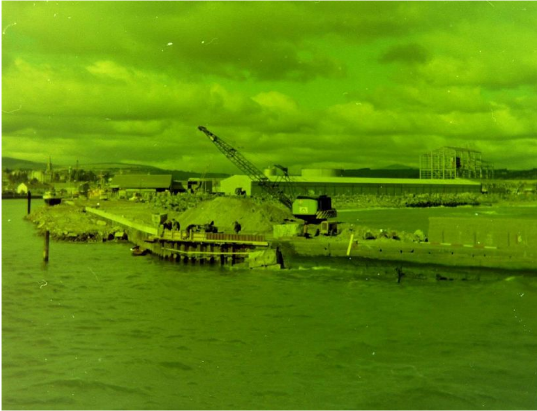
Photograph 6: View of harbour area facing north west showing restoration of the north pier in the foreground and construction of the Arklow Gypsum Ltd. Wallboard Factory and the adjacent IFI tank farm in the background.
