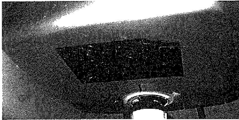
Plate 13 – Felt Patch on the Sink in the Administration Block
