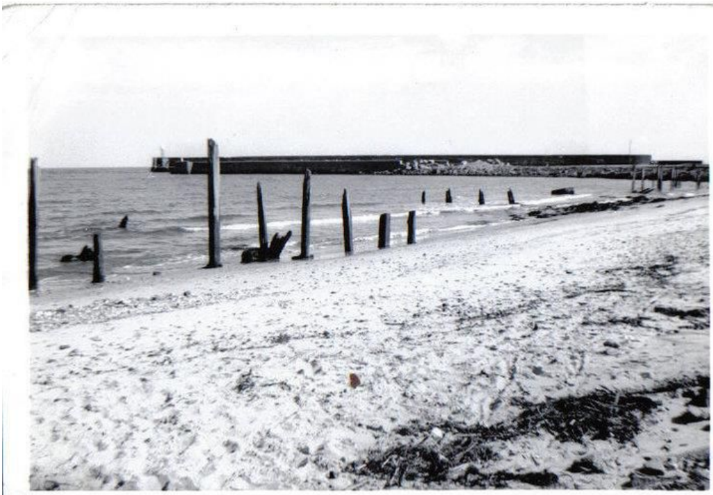
Photograph 5: Coastal erosion protection on beach down from the site, unknown date. View facing south.
