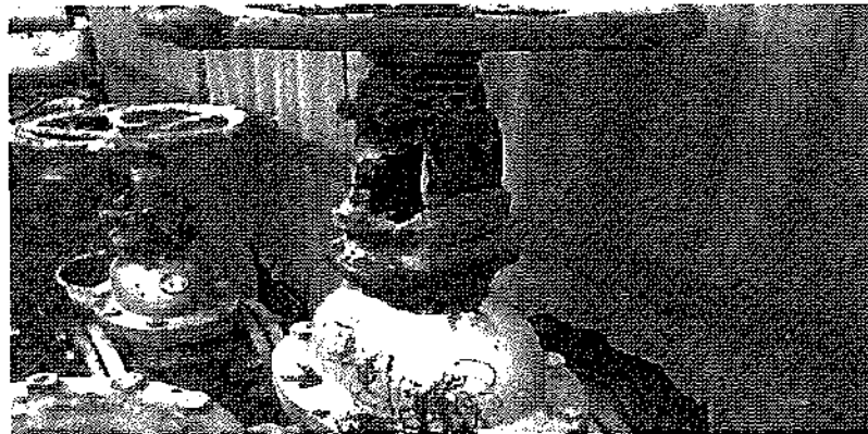
Plate 14 – Webbing on Valve beside the Insulated Tank
