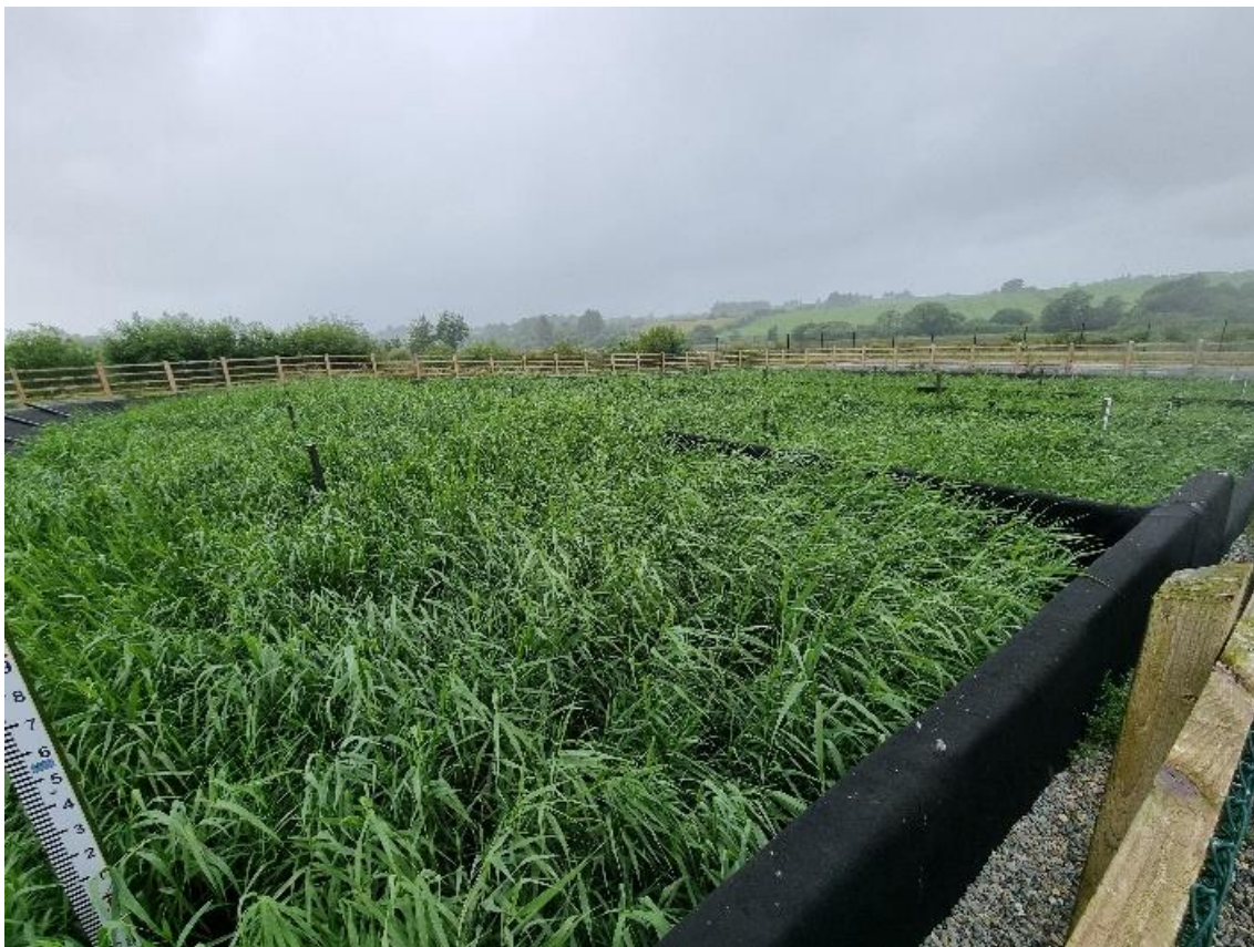
Sludge Drying Reedbeds at Boherbue WWTW, Co. Cork
